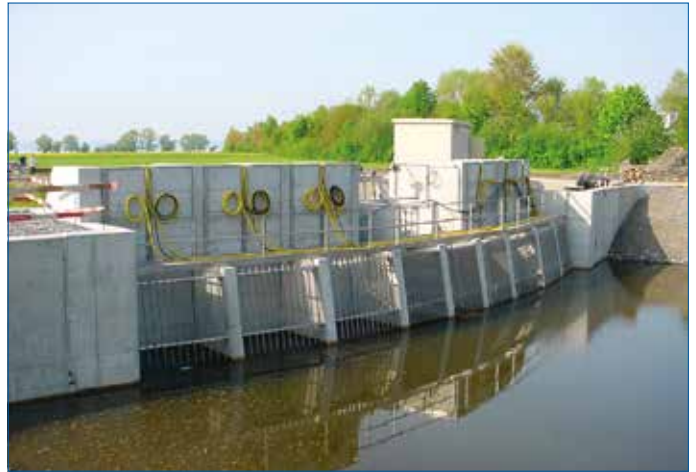
Fig. 65: Coarse screens upstream of an Amacan pumping station (water abstraction from a river)
