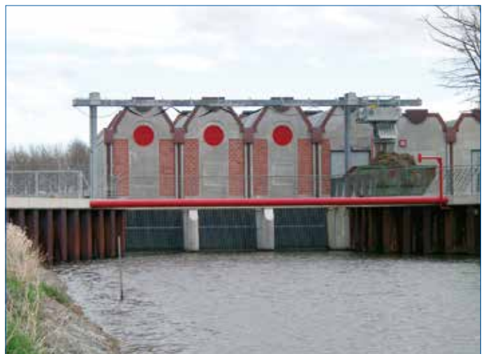
Fig. 73: Pumping station with automatic screens
