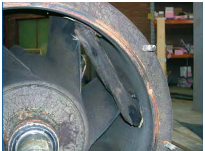
Fig. 72: Wood inside the diffuser casing of an Amacan pump
